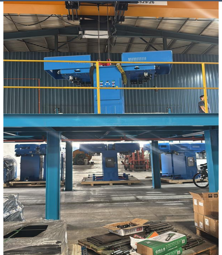
Figure #3 New up-casting line supporting the new copper furnace
